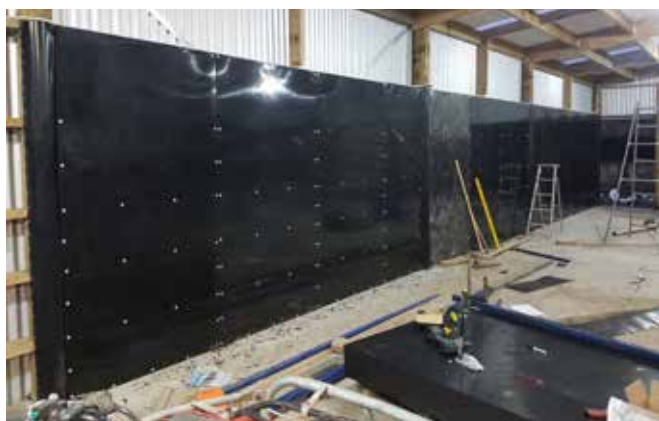
PLASTIC FANTASTIC: The walls are lined with 9ml plastic ply, made from recycled balage wrap, and attached to the steel frame with counter-sunk screws. The plastic walls cost about $19000, almost double the cost of timber ply, but the flipside of the investment is no splintering and damage or touch-up painting.
